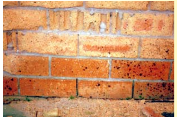
Brick work showing signs of salinity damage and accumulation of brick 'grains' at the base of the wall.
