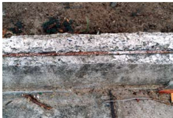
Rust formation exerts physical pressure on the surrounding concrete and leads to weakening of the reinforcement steel.
