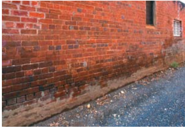
A building with wet 'tide' mark ( dark bricks ) showing the height of the rising damp.
