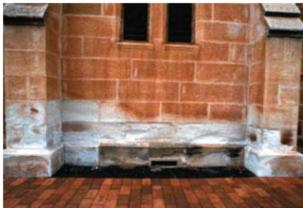
A sandstone church showing signs of salt and water damage.
