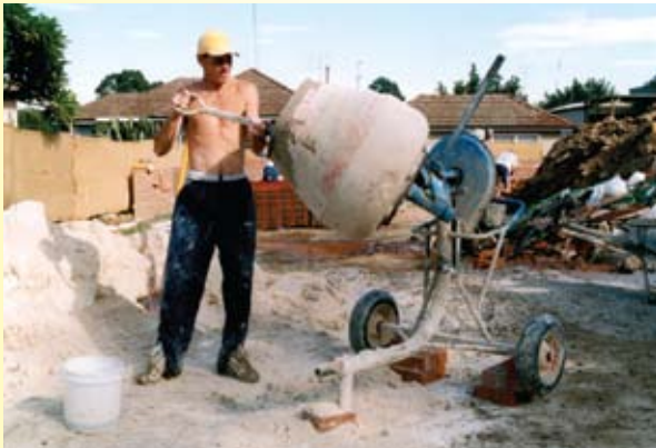
Larger quantities of concrete are delivered to the building site while smaller amounts and cement based mortars and renders are often mixed on site.
