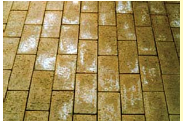
New pavers laid on unwashed sand.
