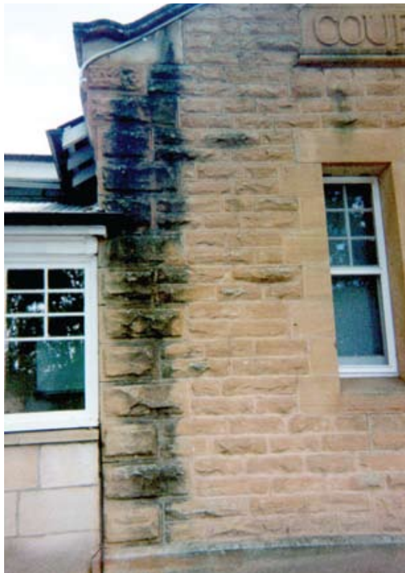
Courthouse showing symptoms of falling damp possibly from a blocked gutter.
