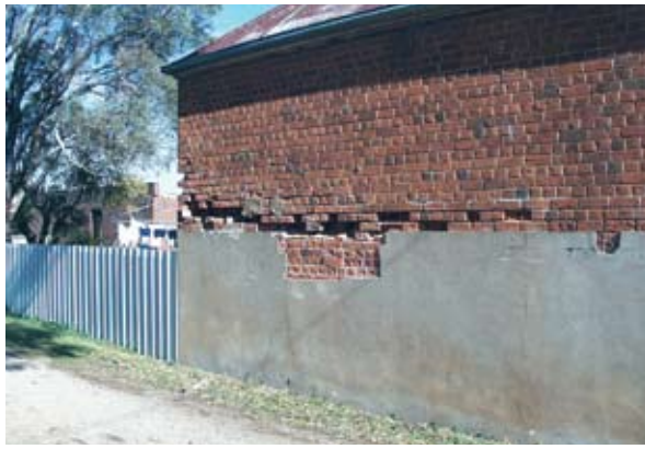
A render with low permeability may reduce evaporation so more water is available to travel up the wall. In this photo, evaporation is occurring just above the top of the render, concentrating salts and resulting in the crumbling of the brickwork.
