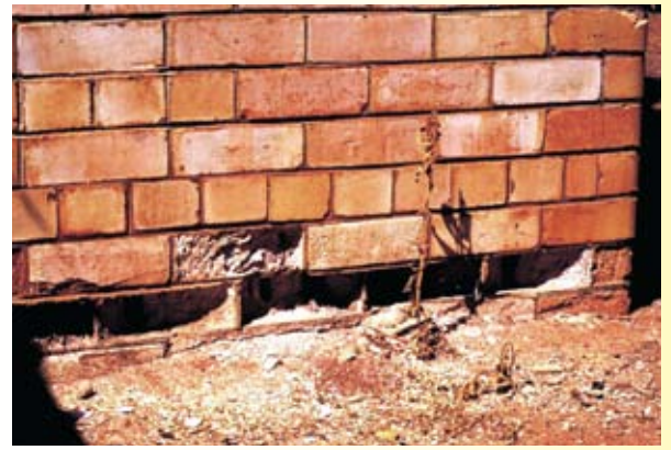
Bricks showing symptoms of salinity damage while the mortar in this case, is slightly more resistant to the physical forces exerted by the salts.
