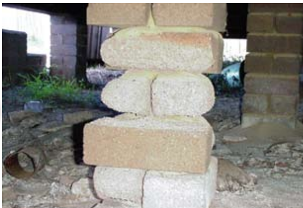
Bricks that have crumbled grain by grain as a result of salt hydration and crystallisation.
