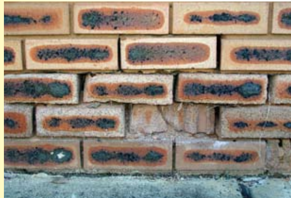
Damage limited to the area below the damp proof course.
