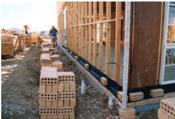
This installation of a polyethylene damp proof course is unlikely to comply with the deemed to satisfy provisions regarding height above finished ground level.
