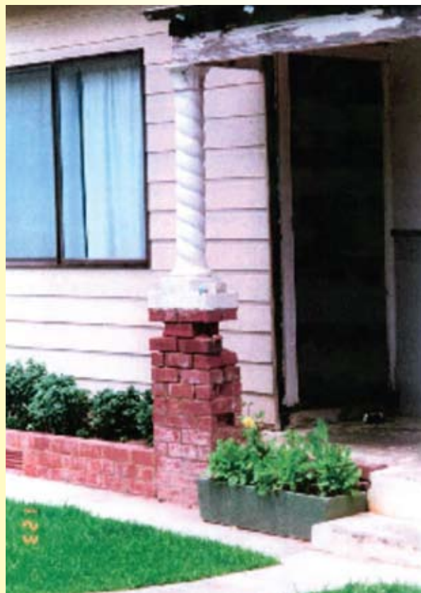
A verandah post showing signs of salt and water damage.
