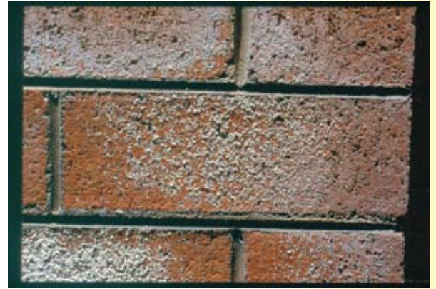
New bricks releasing salts.
