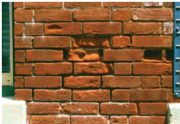
Bricks showing signs of salt and water damage.
