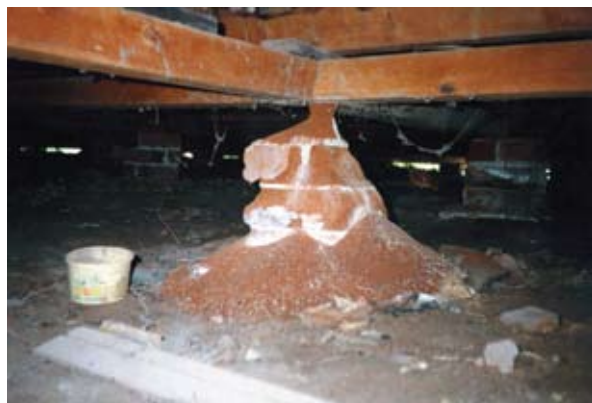
Damage to brick piers discovered during a building inspection.
