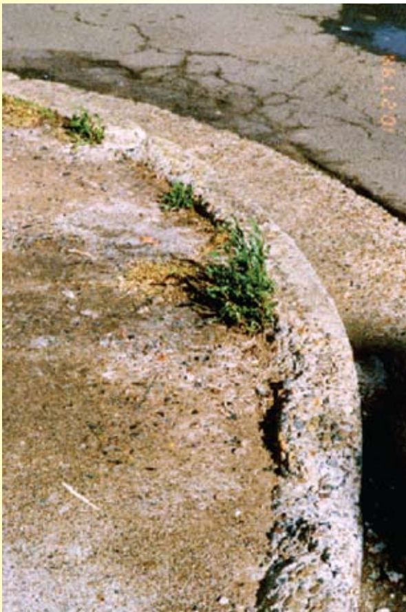
Concrete kerb and gutter affected by sulphates.
