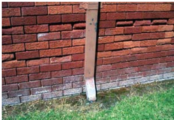
A rusted down pipe allowing rainwater to mobilise salts in the soil.
