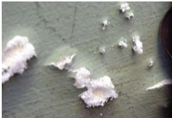
Paintwork blistering due to the accumulation of salts.
